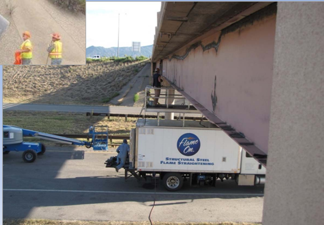
F-06-U, Repaired 9 days later, I-70 Silt Spur over I-70 near Silt Colorado
